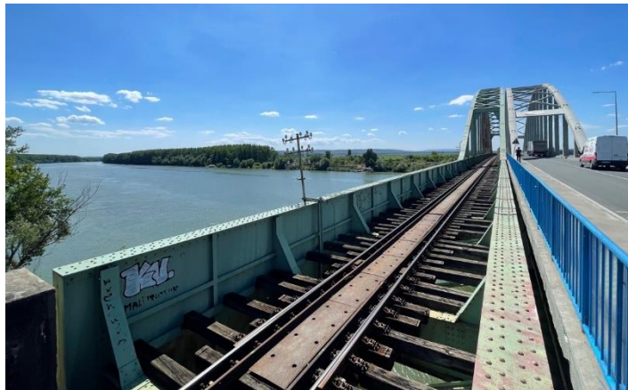
Figure 3: Titel railway bridge across the Tisa River (railway no. 208, chainage 52+279 to 52+679) planned for maintenance as part of the Project (Source: Enova)
