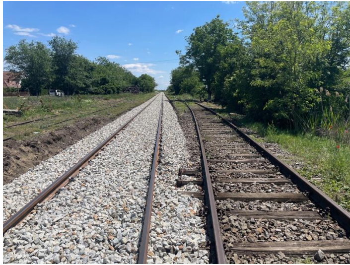
Figure 2: Maintained track at the railway section Lukicevo – Zrenjanin Fabrika (outside of the Project scope) which connects to the railway no. 208 which is part of the Project (Source: Enova)
